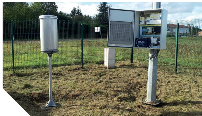
Station de captation
